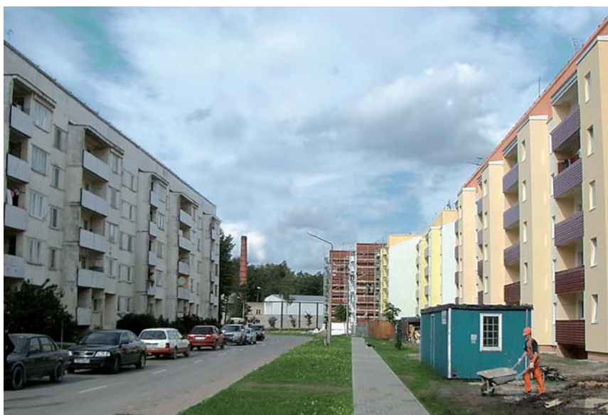
Broceni, Saldus region: Conclusion of the renovation work in Skolas Street in autumn 2004
